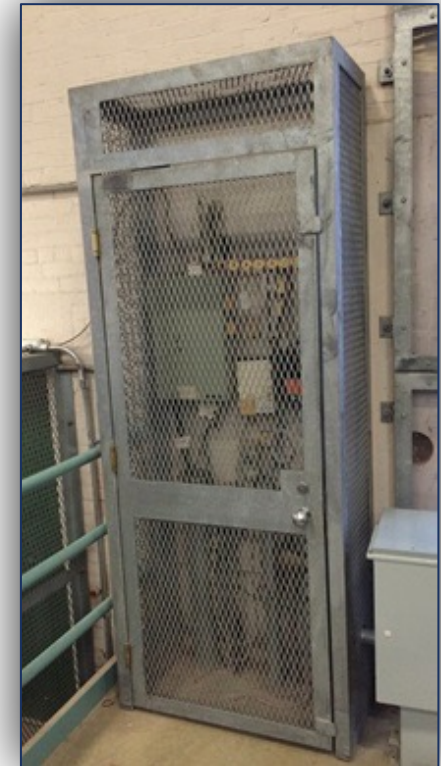
Cage protecting telecom demarc
